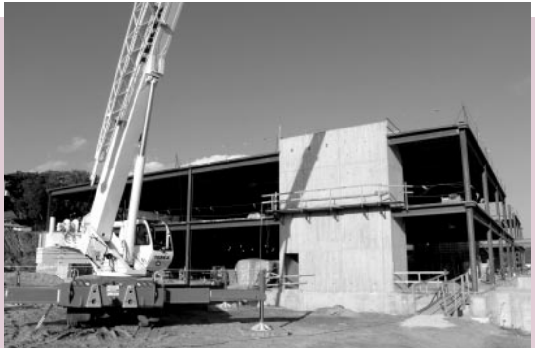
Construction is underway on Franciscan Skemp's new Onalaska clinic. When the 96,000 square foot facility opens in mid-2006, it will house a practice unlike any other in the region.
